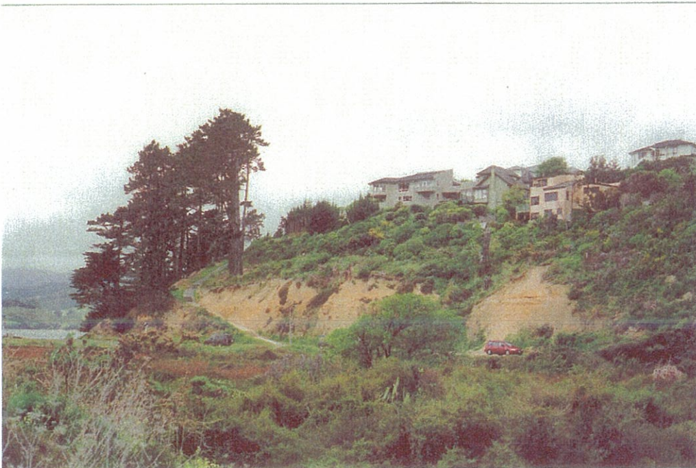
Exposed and eroding surfaces need a vegetation cover.
