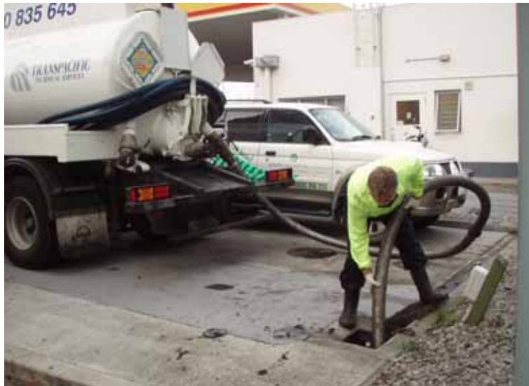
A stormwater sump being cleaned out after a hydrocarbon spill at Shell Thorndon
