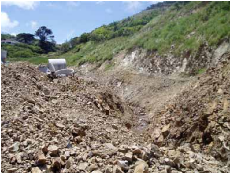
Poor sediment controls at Kiwi Point Quarry
