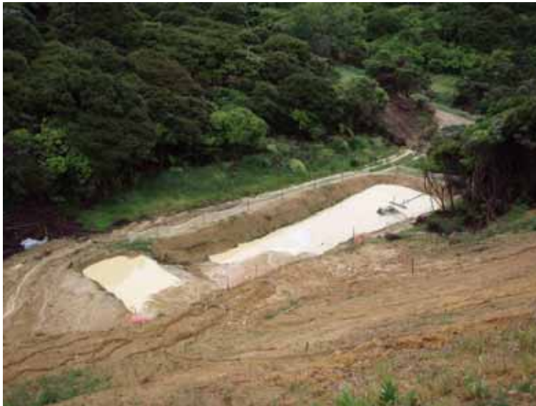
Sediment run-off at Staithes Drive development
