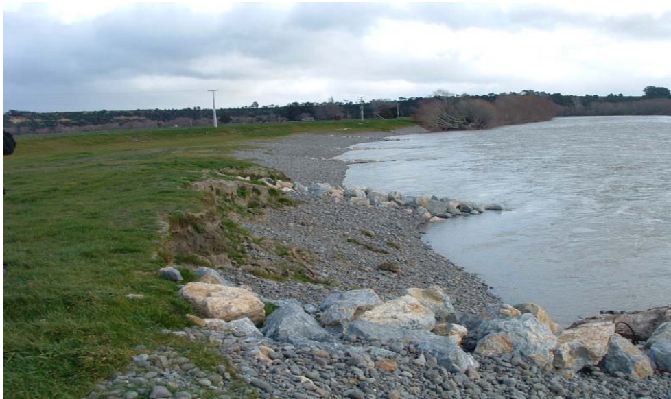
Picture 4: Series of rock groynes on the Guscott's property
