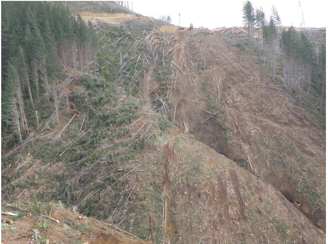
The view from the bulldozer anchoring the haul lines looking back towards the hauler and the skid
