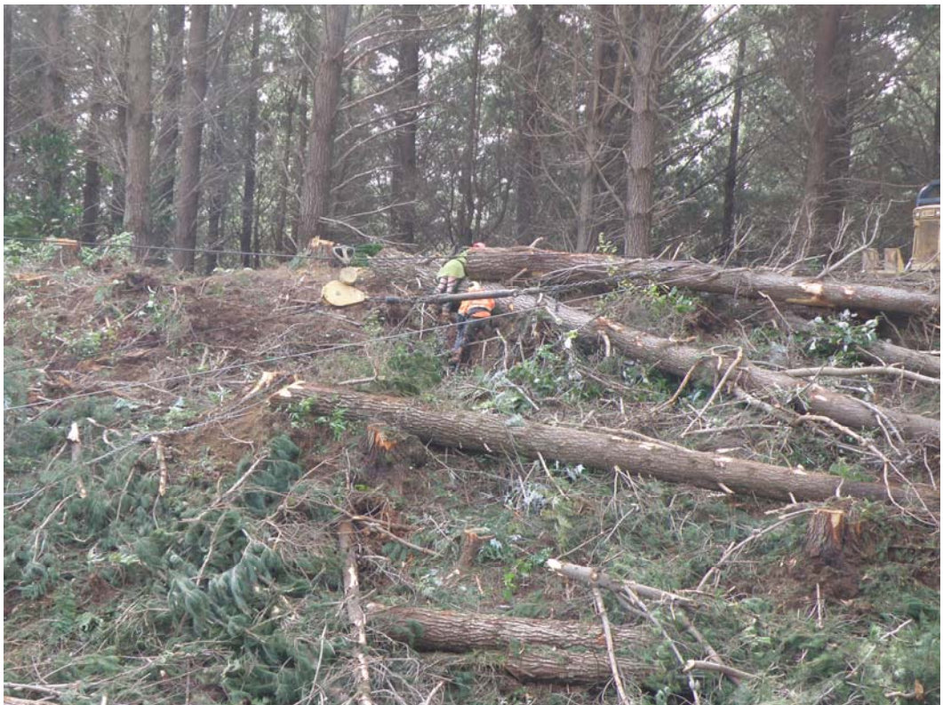
The breaker outs coupling log onto the haul lines, with the bulldozer as an anchor in the background
