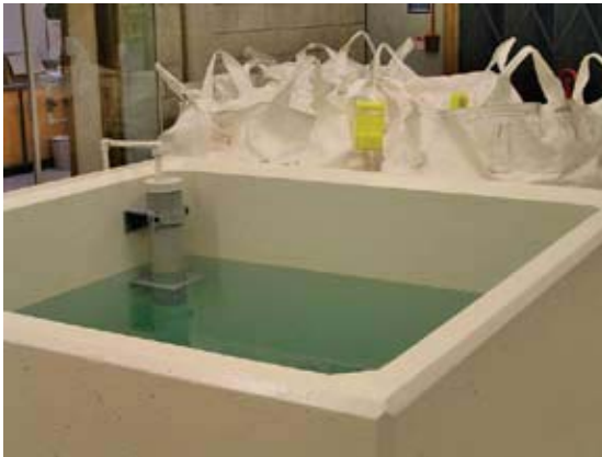
Generating chlorine from saltwater at Te Marua will save an estimated $80,000 annually. This picture shows the hypochlorite plant's brine tank
