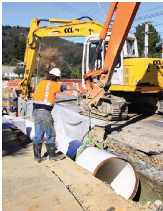
Diggers lift a new section of the Wainuiomata water main into place
