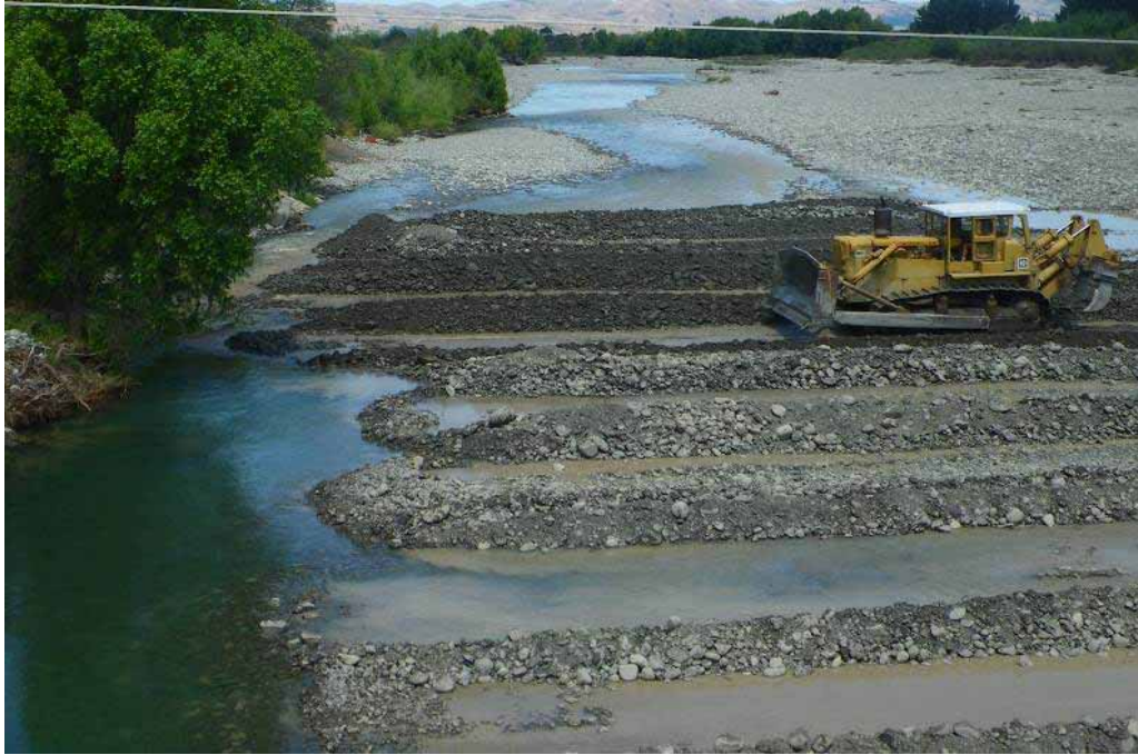
Figure 6.3 A bulldozer realigning a section of the Waingawa River channel to reduce erosion that is occurring along the left bank
