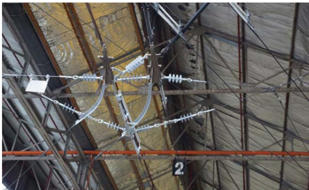
Special works in Kilbirnie bus barn, with polymer insulators
