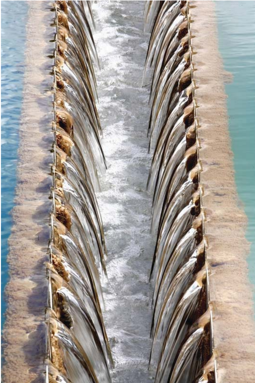
Part of a clarifier at the Te Marua Water Treatment Plant
