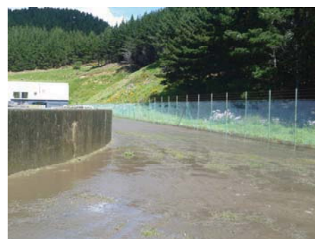
Wastewater overflowing the aeration basin and ponding on the ground at PCC WWTP, before flowing into the stormwater channel, stream and into the CMA
