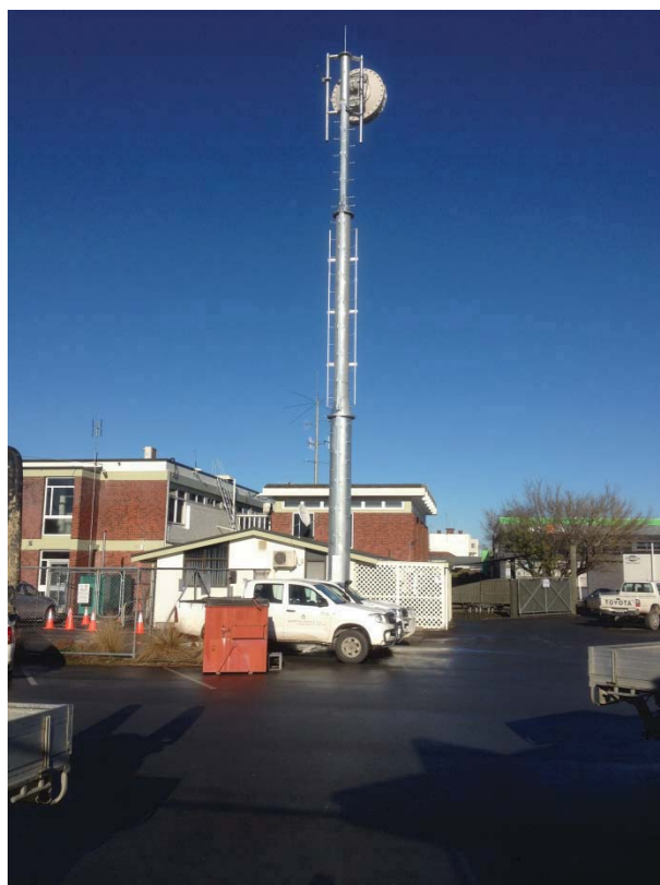
Recently installed Hawan Mast at Masterton office
