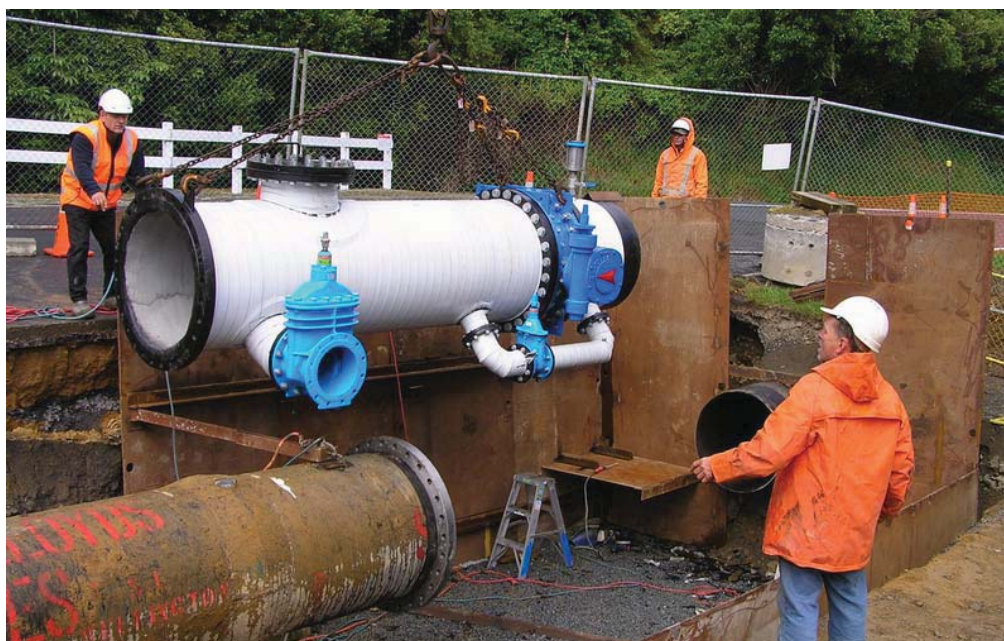
A new line valve at Mangaroa
