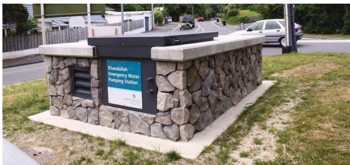
The recently commissioned Khandallah Emergency Water Pumping Station
