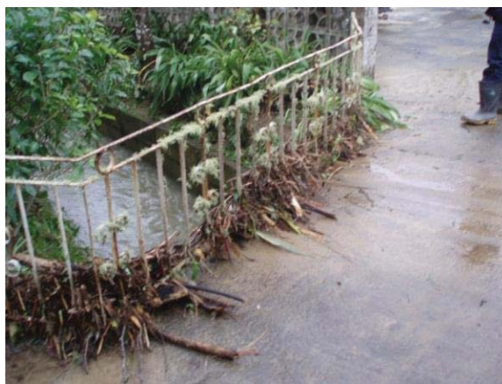
Figure20: Debris from overtopping of a culvert in flood
