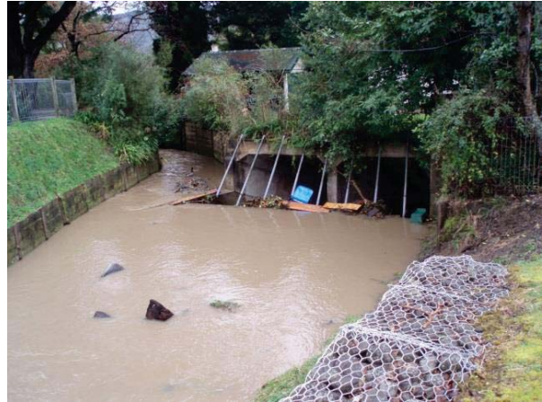
Figure 8 - Blockage forming at bypass intake
