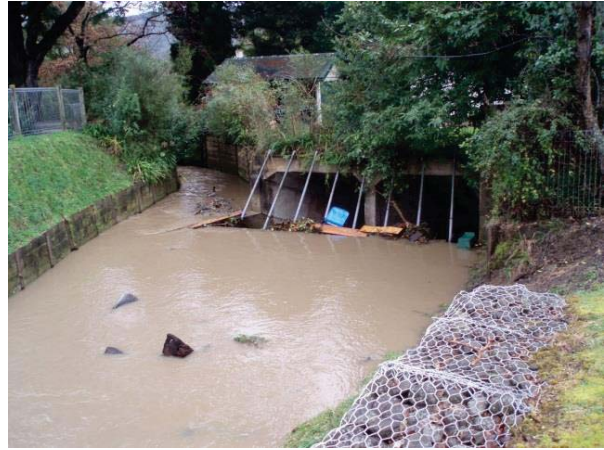
Figure 8 - Blockage forming at bypass intake
