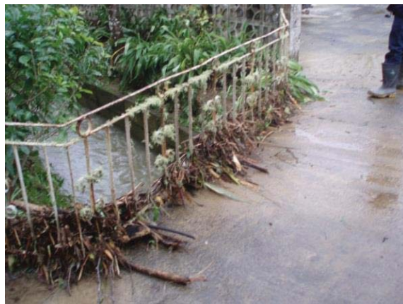
Figure20: Debris from overtopping of a culvert in flood
