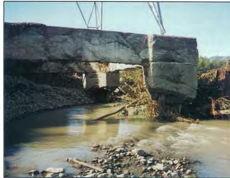
PHOTOGRAPH 7: UNDERMINED LEGS OF THE TRANSPOWER PYLON IN JIM COOK PARK
