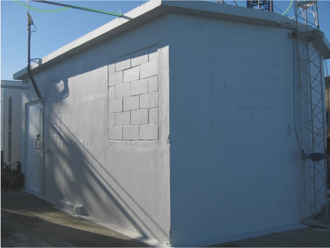
Fig. 23. The WWII radar building from the south-west with the blocked-in bow window and other window apertures.
