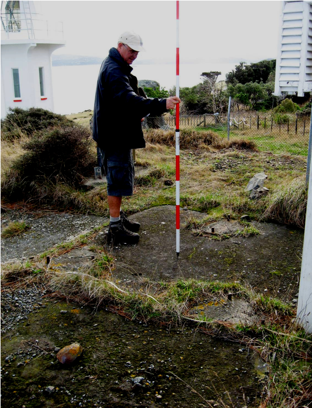
Fig. 21. The radial arrangement of bolts for the brackets holding the signal mast.
