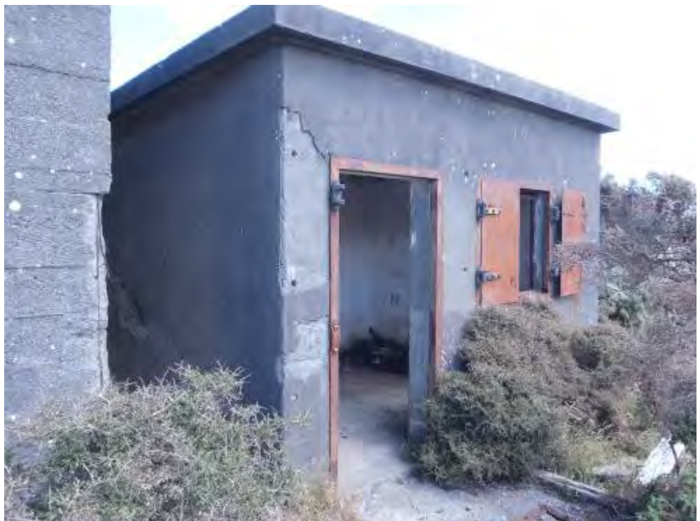
Figure 30: The wireless room. The reinforced concrete walls were rendered on the outside. The shutters are still in place and at the bottom of this photograph there is visible a small portion of the door which currently rests on the ground in front of the building.
