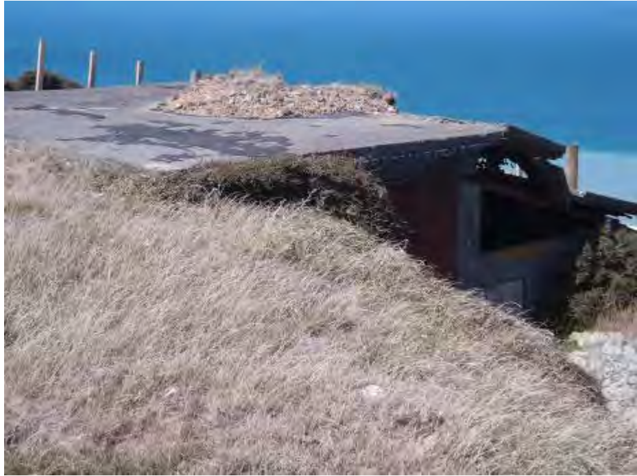
Figure 27: The observation post, built of reinforced concrete. Inside is the concrete foundation of what might have been a range finder or telescope. This building retains part of its camouflage (a layer of earth and vegetation visible on its roof) but the cantilevered roof over the viewing slit has collapsed. The path that has been constructed to allow entry to the building is shown to the right of the photograph
