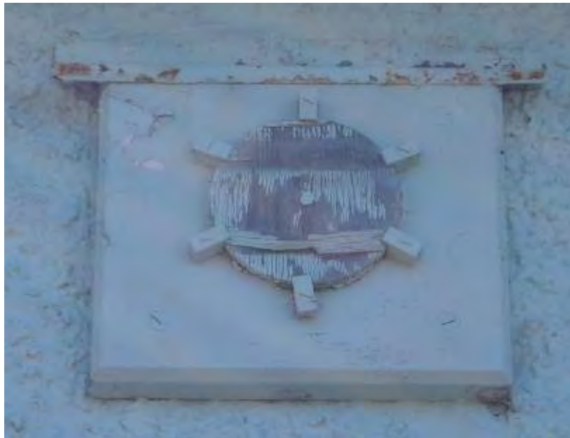
Figure 18: Close up of plaque attached to the front elevation of the diesel generator building.
