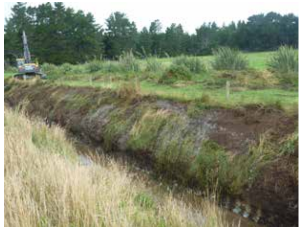
Poor practice: The vegetation has been scraped off the bank with the bucket.
