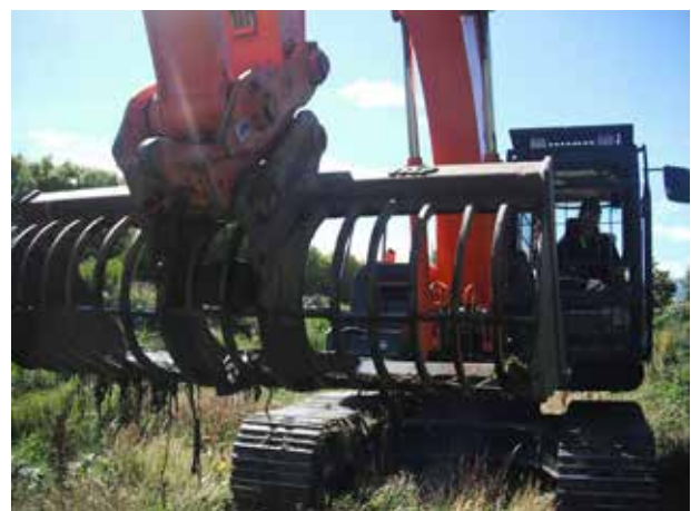
Example of excavators with weed rakes attached. Fish are able to swim through the large gaps and are less likely to be caught than if a standard bucket was used.
