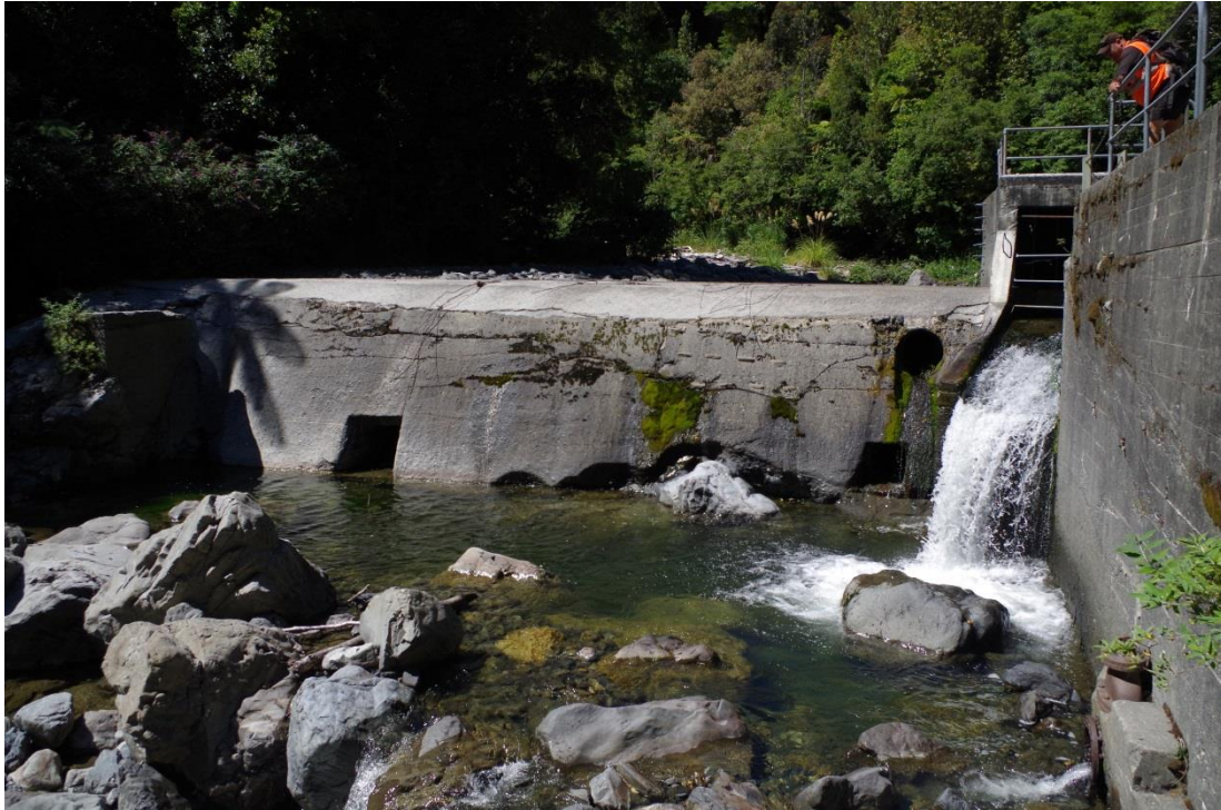
Orongorongo water supply main weir viewed from downstream to the northwest (Dodd, 2015)
