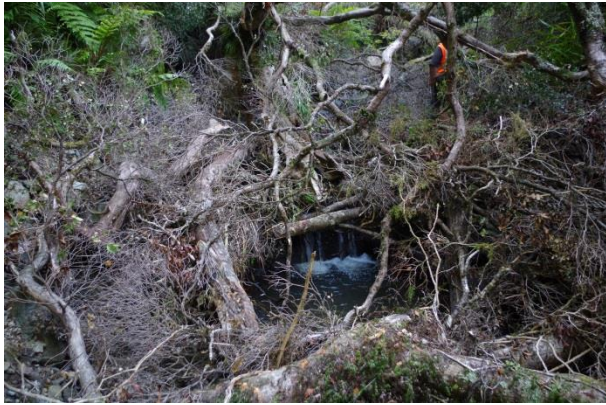
Telephone creek weir and intake viewed from the south. Obscured by fallen trees
