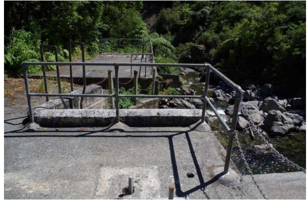
Main weir looking SE across the top of the intake structures on the true left
