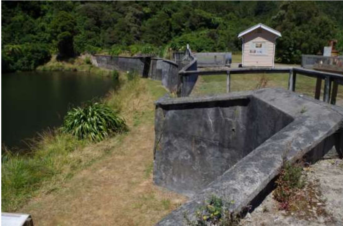
Wainuiomata water works dam, looking southeast along the face of the dam (Dodd, 2015)
