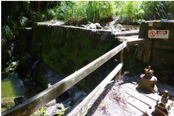
Big Huia intake viewed from the track adjacent to the intake structure
