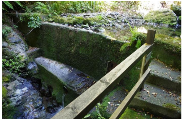
Little Huia intake viewed from the track adjacent to the intake structure
