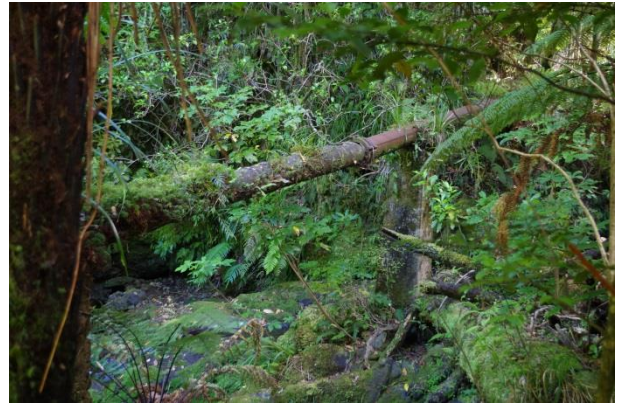
Telephone creek water supply pipe on concrete supports in the stream bed to the south of the weir and intake
