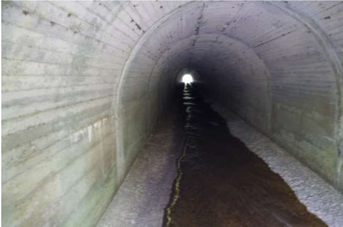
Inside of the stream diversion tunnel, looking southeast from northwestern end (Dodd, 2015).
