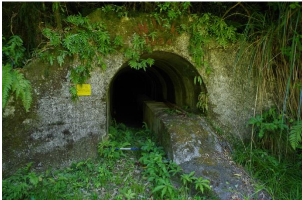
Short tunnel, eastern portal, with water supply pipe leading into concrete abutment on the right hand side
