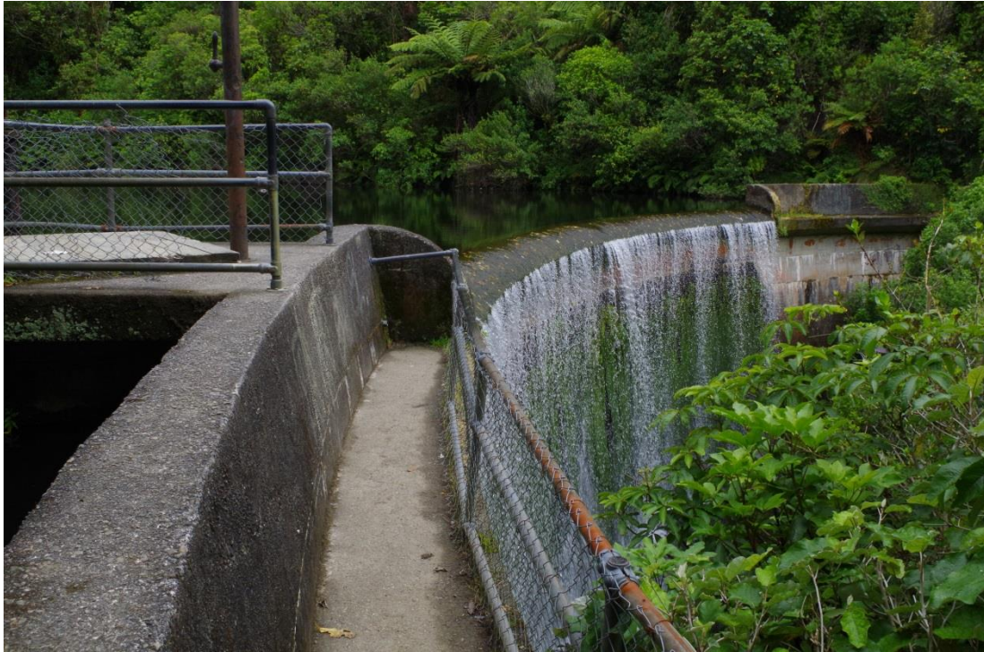
Main dam, looking across crest of dam past intake valves towards spillway (Dodd, 2015)
