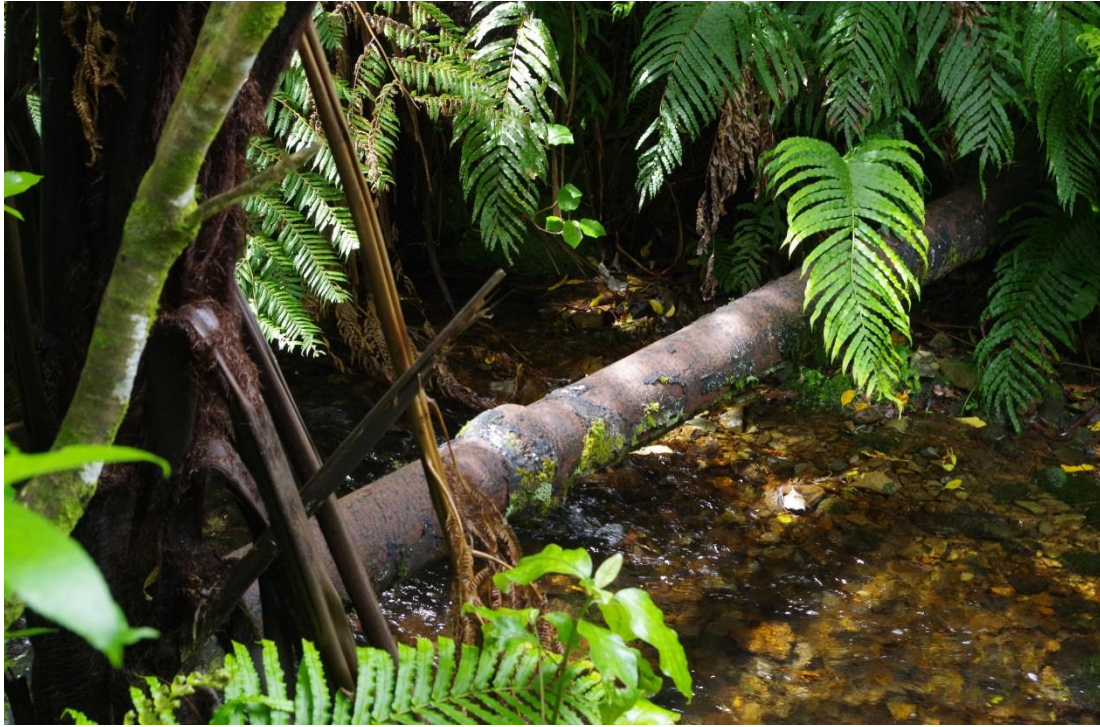
Disconnected sections of water supply pipe in stream south of dam (Dodd, 2015)
