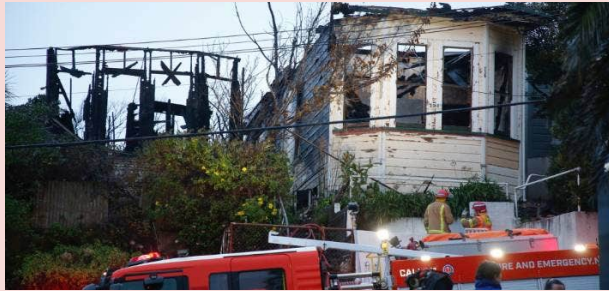
Above: Aftermath of the fire at Hanson Street.
