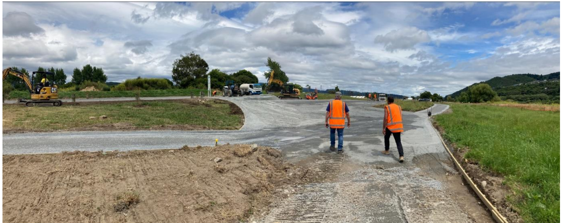
Figure 2: Poets Park central carpark area (accommodates future toilet block) and trail under construction
