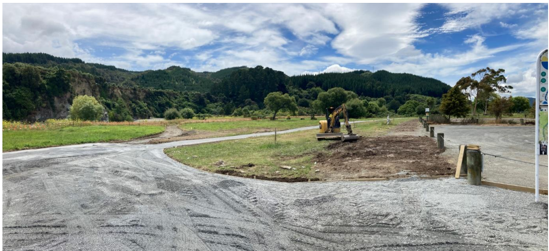
Figure 3: Poets Park - Old track being removed and turned back to grass. Existing track down to river being upgraded also.
