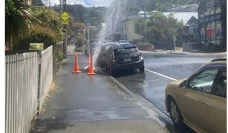
The major burst in Te Aro, which meant our crews had to stop proactive leak repair work in Brooklyn in order to respond to this.
