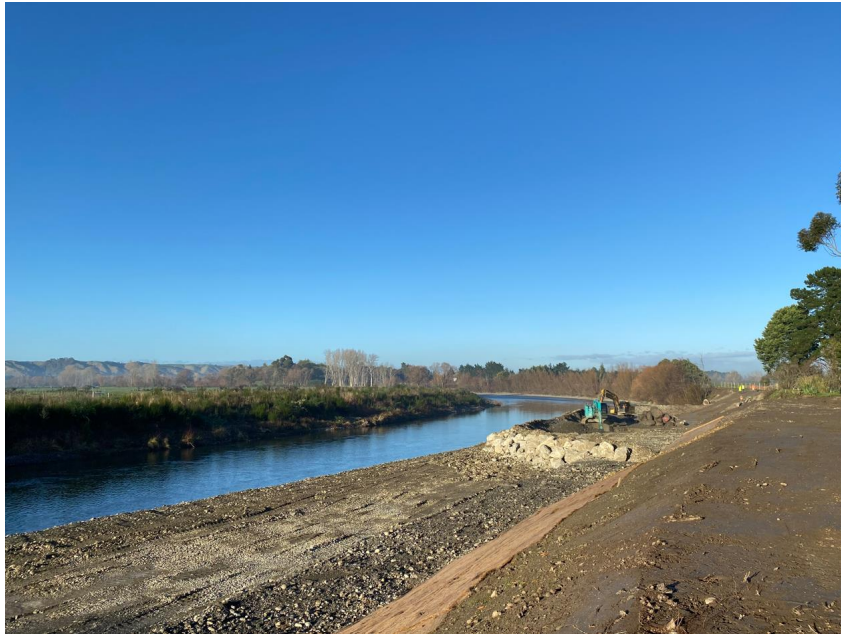
Figure 10: Stage two (Ruamāhanga River) – Construction of the rock revetment continues within the Ruamāhanga River
