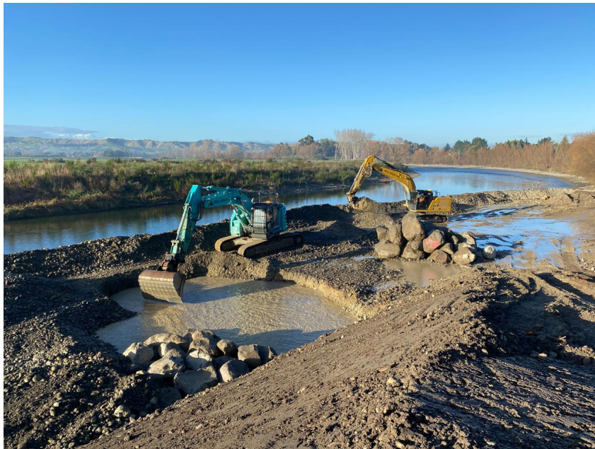
Figure 11: Stage two (Ruamāhanga River) – Excavation of the rock revetment within the Ruamāhanga River (the excavation is banded from the Ruamāhanga River and is not within the flow of the river)
