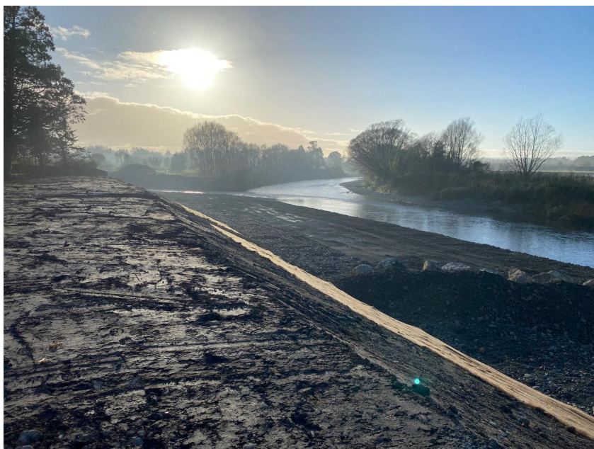
Figure 12: Stage two (Ruamāhanga River) – A section of the rock revetment within the Ruamāhanga River is completed. The temporary bunding has been retreated. This photo overlooks the confluence of the Waipoua and Ruamāhanga Rivers
