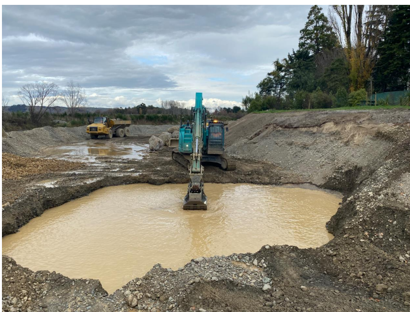
Figure 7: Stage two (Waipoua River) – Excavation of the rock revetment within the Waipoua River (the excavation is bunded from the Waipoua River and is not within the flow of the river)
