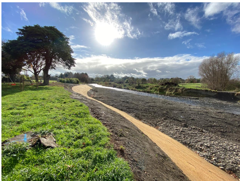
Figure 8: Stage two (Waipoua River) – Rock groyne and rock revetment completion within the Waipoua River. Coconut matting has been installed to the battered river bank above the rock revetment
