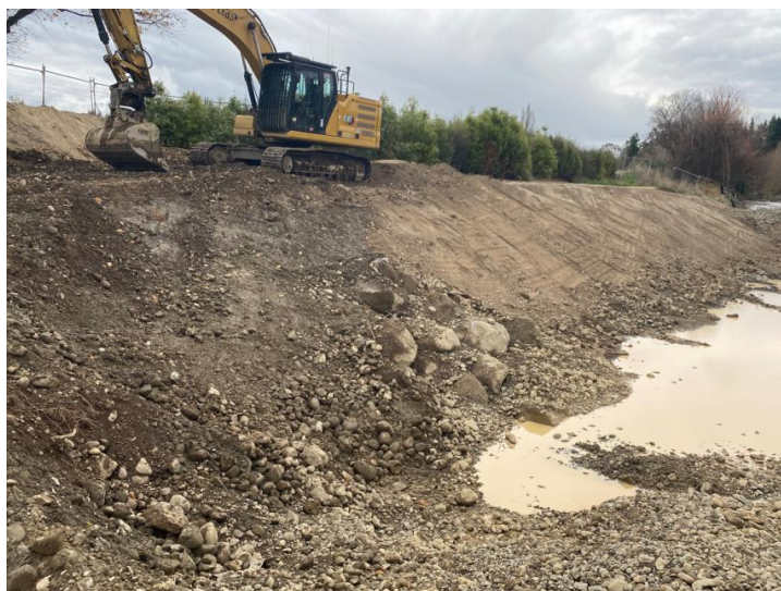
Figure 6: Stage two (Waipoua River) – 1,000 tonne rock groyne completed within the Waipoua River
