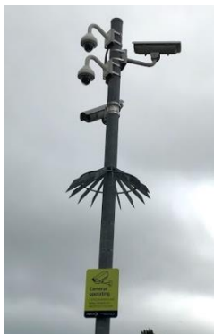
Figure 44: Station CCTV cameras
