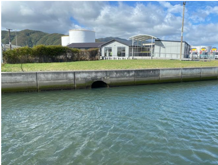
Figure 13: Location of the Seaview Wastewater Treatment Plant wastewater discharge to the Waiwhetū Stream.
